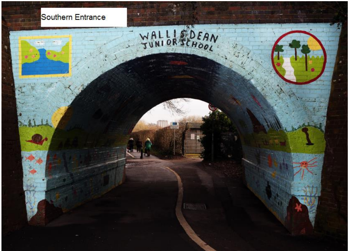
Worn paint on current mural
